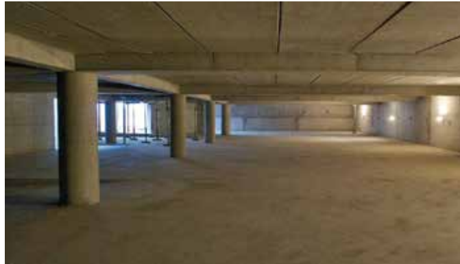
Fig. 6: The parking-level floors were constructed using precast prestressed slabs on cast-in-place beams
