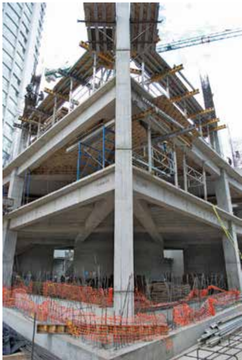
Fig. 5: View of “back” of tower showing the 30 x 20 m (98 x 66 ft) column-free interior space (for scale, see workers inside). The special A-grid beam arrangement that allowed the elimination of all the interior columns is also visible in the exposed ceiling
