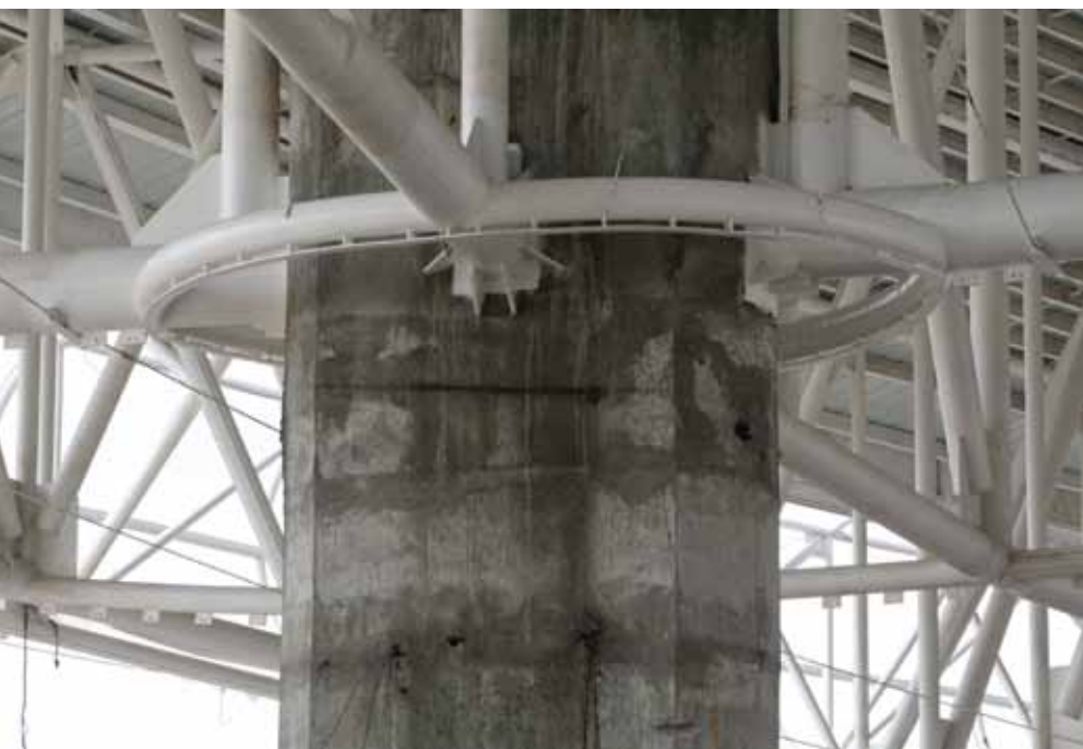
Fig. 6: Connection detail between a macrocolumn and main radial roof truss and circumferential roof trusses (photo courtesy of Juan Pablo Beas)
