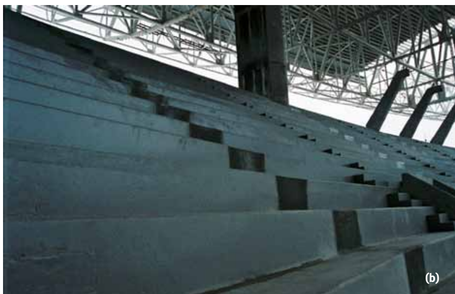
Fig. 7: Precast-prestressed seating elements were produced on site: (a) units included exposed passive reinforcement for subsequent embedment in continuity joints at raker beams; and (b) the continuity joints for the precast seating units (dark concrete) help to avoid leakage from rain and drinks, and they reduce crowd vibration issues, both common problems with simply supported seating units
