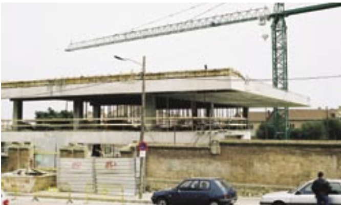
Fig. 7: Partial view of the finished structure showing a long cantilever roof at Block 1
